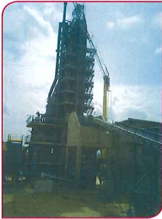
Right: The SIC HPK lime kiln installed for Carrieres et Chaux du Mali in Mali.
