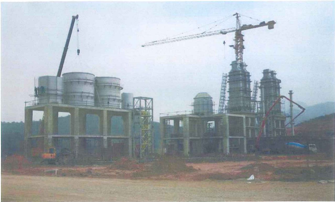
SIC has been contracted to construct a new lime plant near Ha Long Bay.
