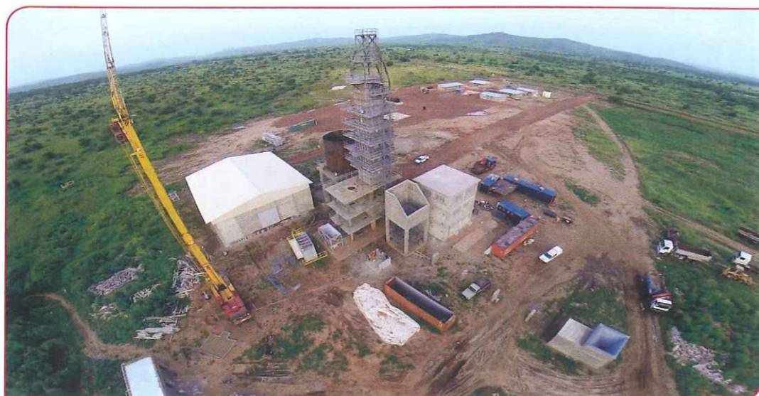
Right: Work is ongoing at the Carrières et Chaux du Mali plant near Bamako.
