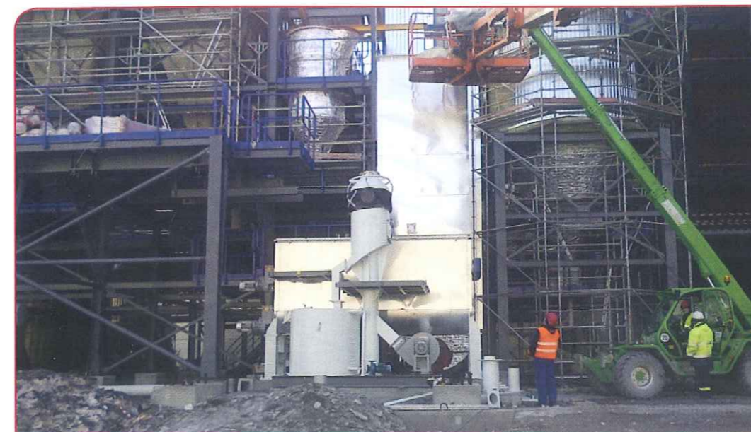
Left: Installation of the Vantaa Energy lime hydrator. The slaked lime produced will be used to neutralise exhaust gases from the company's waste incinerator.
